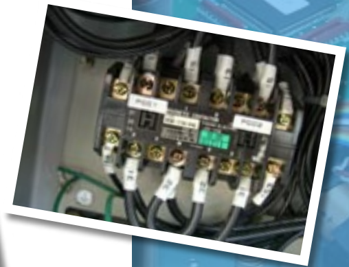
No faults or corrosion found in the phase correction contactor
