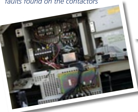
No deterioration or corrosion faults found on the contactors
