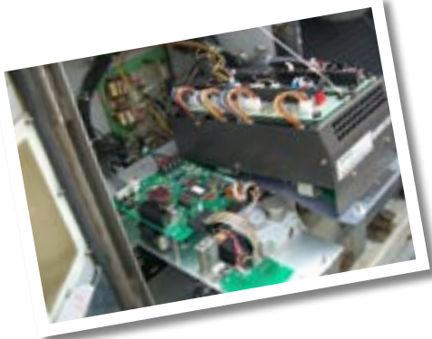
The electric components in the controller box No deterioration or fault effecting operation
