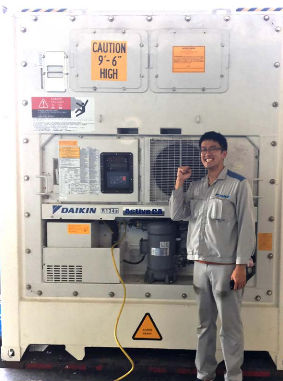
Left: Daikin's retrofitting trials in September showed that units could be fitted with the latest Daikin CA units in under three hours, making it a fast and cost-effective refrigeration solution.
